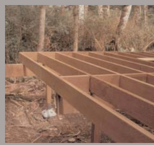
For some structures, dead load may be applied before driving pins, or applying caps.
